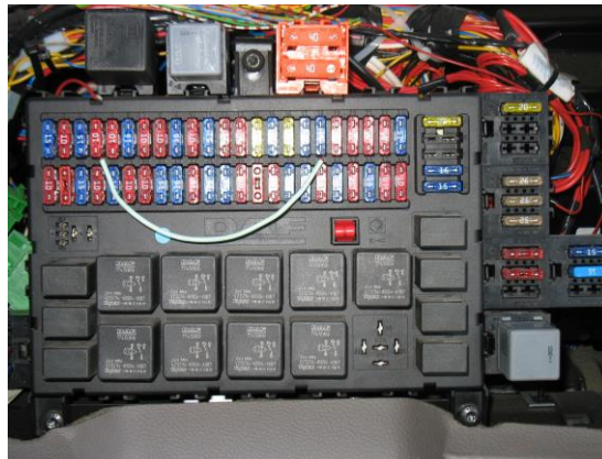
Figure 4 Fire cause: illegal bridging of fuses
