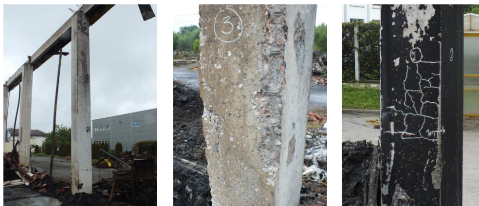
Figure 4 – Characteristic defects and damages of concrete elements in “Uradi Sam” caused by fire: Peeling of crumbly concrete along the column edges, visible reinforcement, net-like fissures, change in aggregate colour
