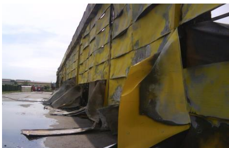
Figure 5 – Deformation of aluminium panels
