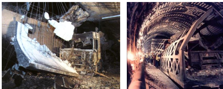
Figure 2 –Damages of secondary tunnel linings caused by explosive spalling of concrete [5,6]
