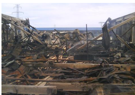
Figure 7 - Collapse of the roof structure in fire
