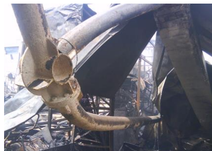
Figure 6 – Collapse of steel pipe
