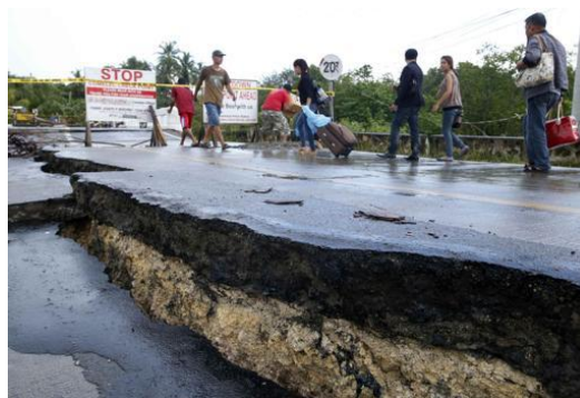
Fig. 21. Surface rupturing due to activation of a fault
