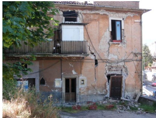
Fig.17. Damaged masonry structure due to the L'Aquila earthquake
