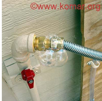
Fig.35. Leakage of gas
