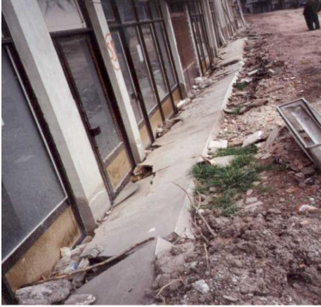
Fig.20a) Sinking due to Adapzari earthquake
