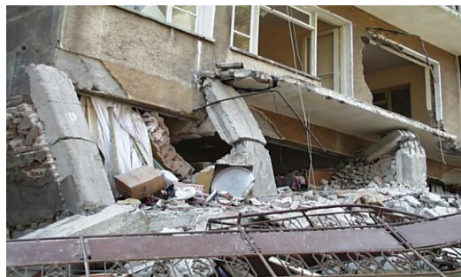
Fig. 32. Voids made during collapse of a building
