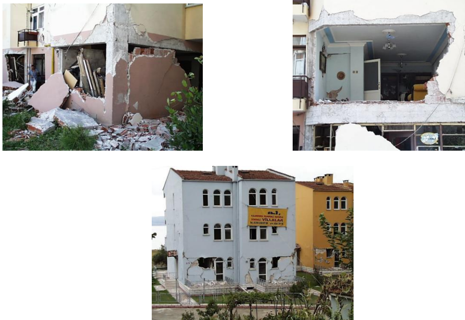
Fig. 13. Damage to non-bearing elements of frame buildings
