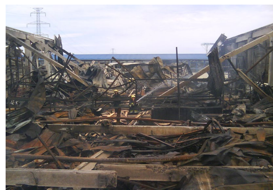
Figure 4. Fire in industry hall-building Uradi Sam in Novi Sad, the collapse of the steel roof structure, 2013. [6]
