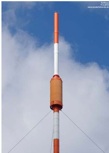
Figure 9. Mast in April 2015 [2]
