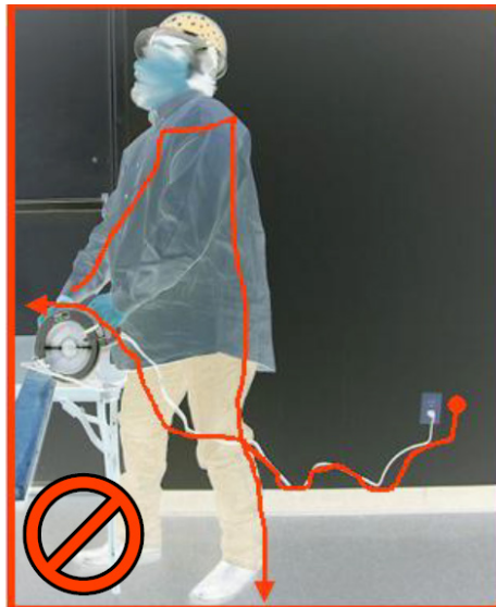
Figure 1. - Worker shocked after a direct contact with the electricity (damaged tool).
