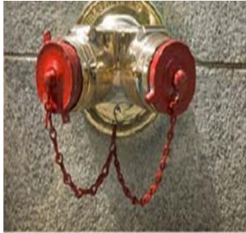
Siamese connection to standpipe
