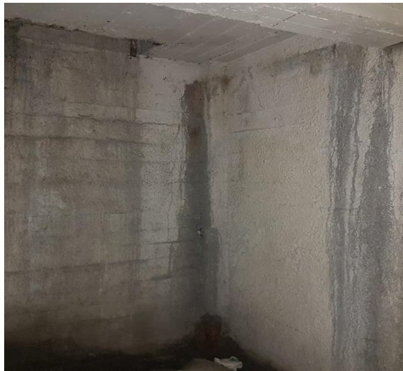
Figure 17– Leaching of lime in concrete
