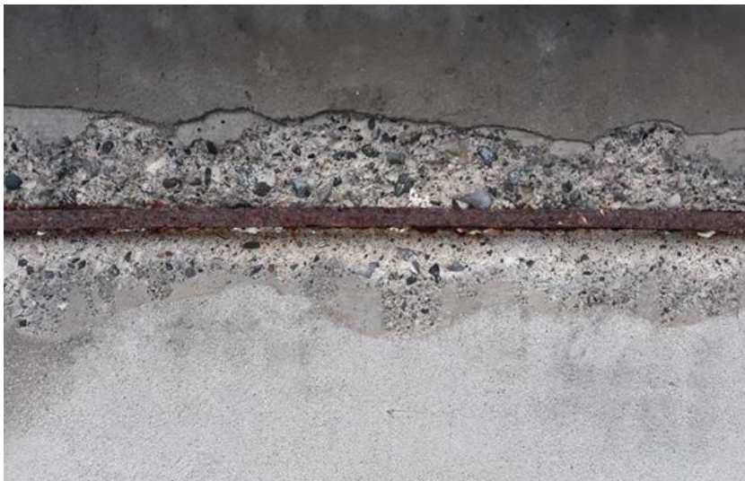
Figure 16– Corrosion in reinforced concrete
