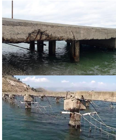
Figure 18– Concrete in sea water
