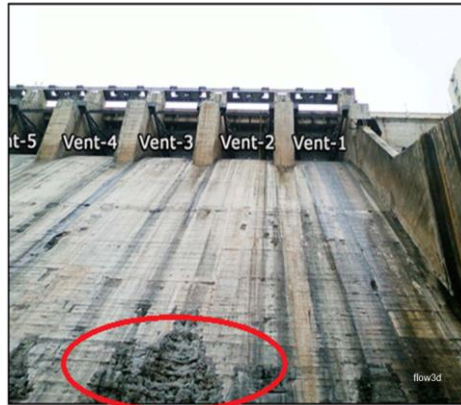
Figure 9– Spillway concrete deteriorated from cavitation
