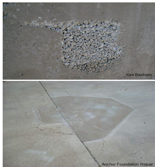
Figure 8– Segregation and patched concrete
