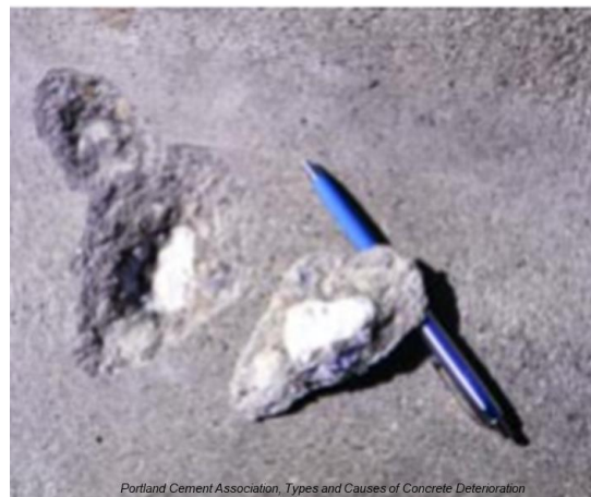
Figure 11– Aggregate expansion in concrete
