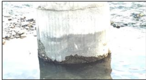
Figure 7– Concrete deteriorated from erosion
