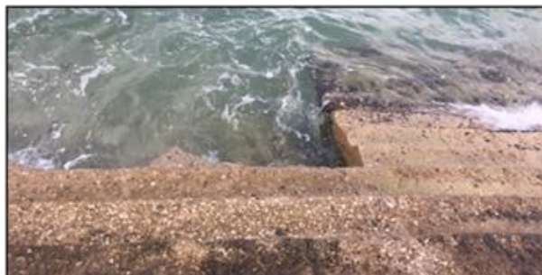
Figure 6 – Erosion of concrete from sea waves
