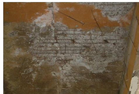
Figure 4: Sloughing off spalling (slab)
