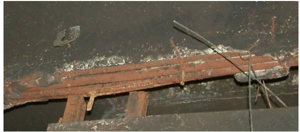
Fig. 16. Characteristic damages of improper reinforced rib due to fire
