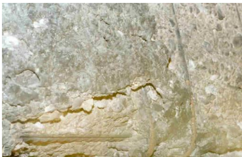
Figure 3: Sloughing off spalling (beam)
