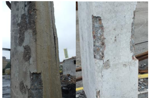
Figure 2: Corner spalling and corner cracks along main reinforcement
