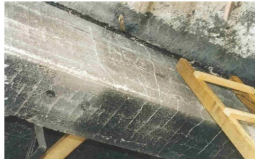
Figure 6: Crazing – mesh like cracks
