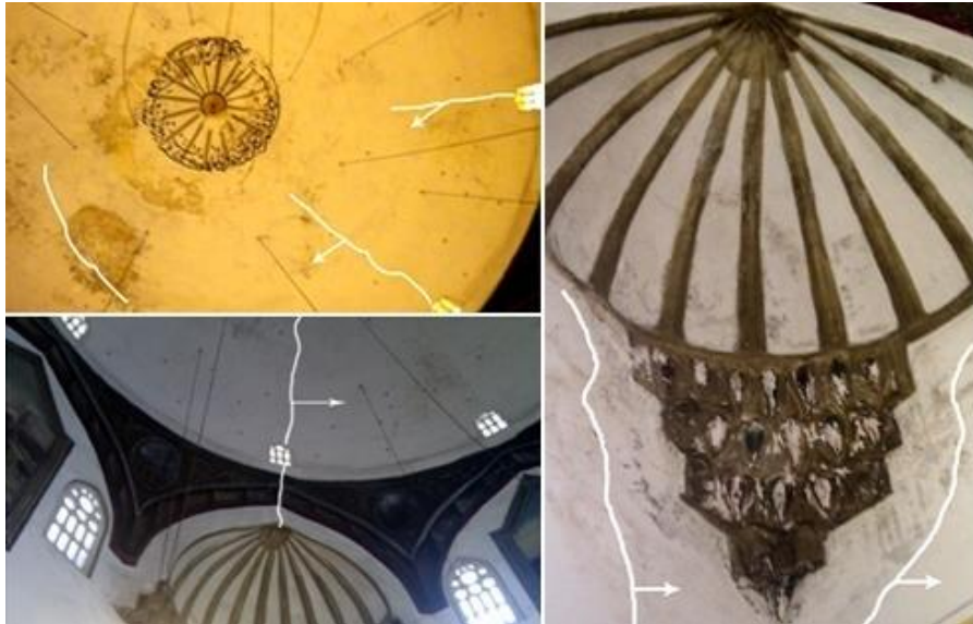
Figure 3 - Cracks in the interior of the dome and pendentives in Mirahor Ilyas Beg Mosque.
