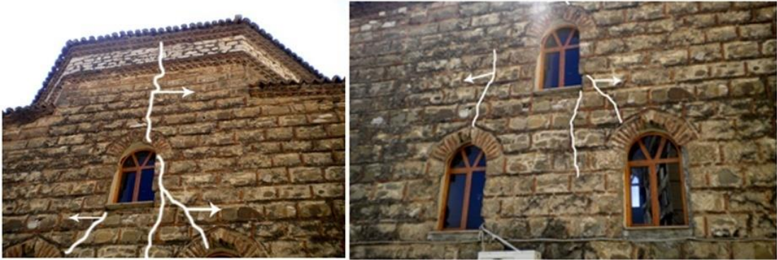
Figure 4 - Propagation of cracks in the load bearing walls, west façade of Naziresha's Mosque
