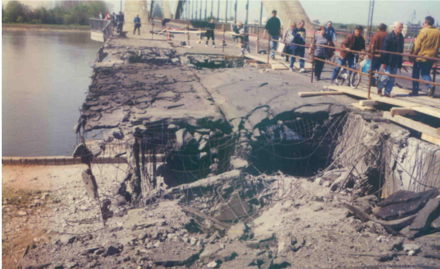
Damaged Deck Structure After the First Attack
