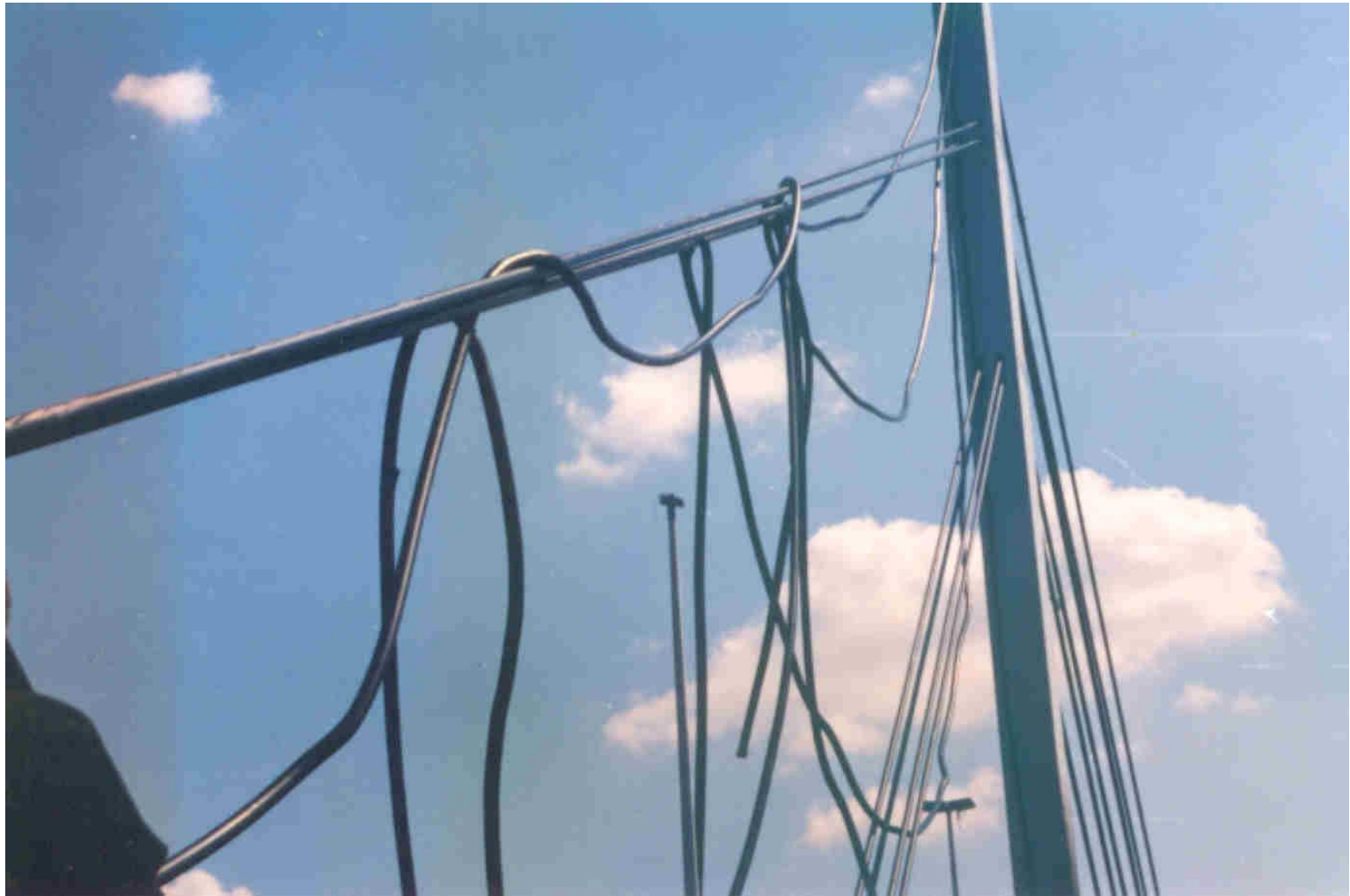
A Detail of the Broken and Damaged Cables
