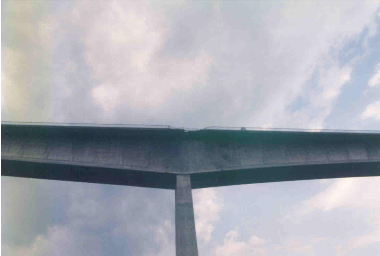
The Damage of the Fence of the Bridge
