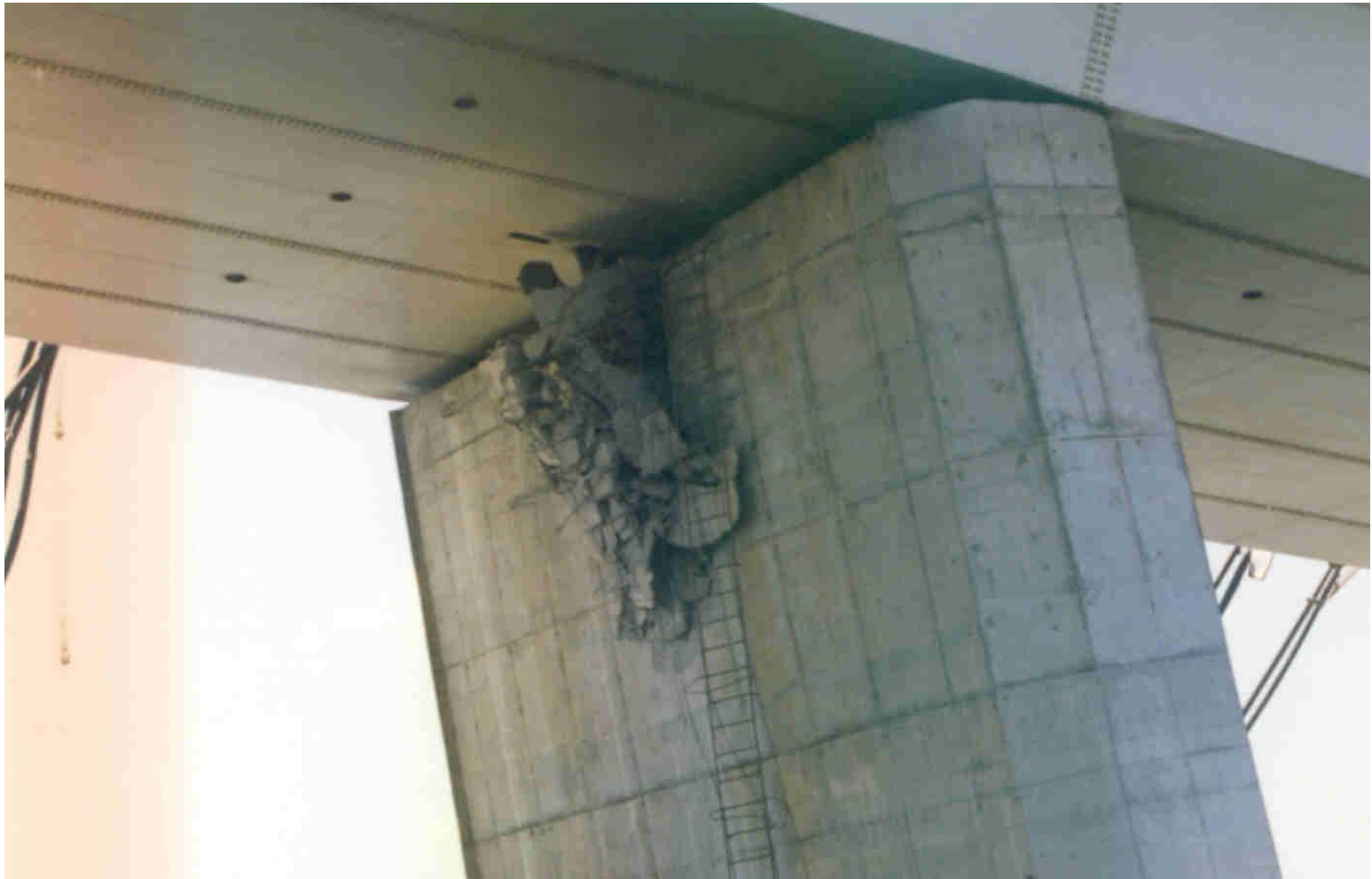
The Damaged Top of the Pier and its Inclination
