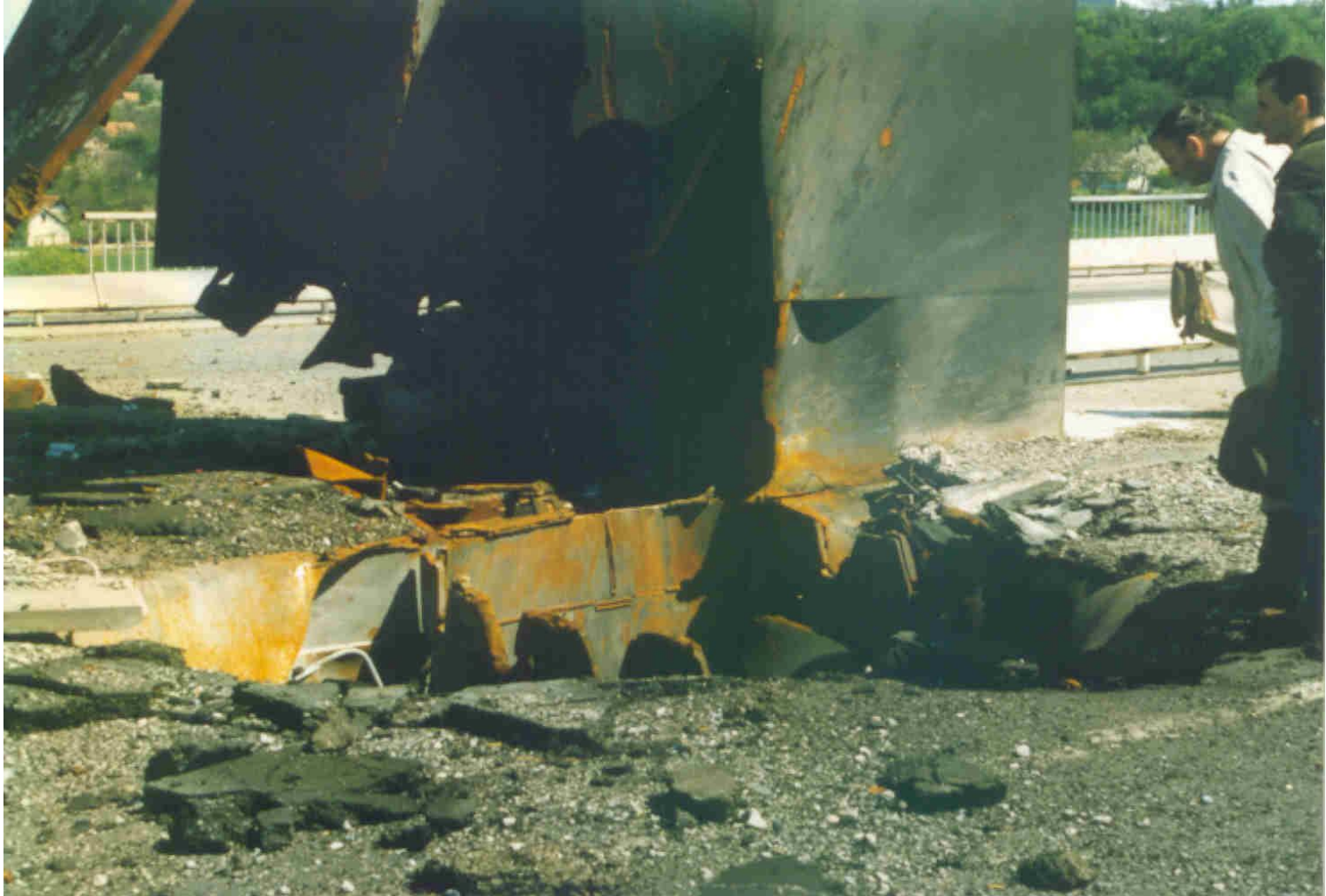
A detail of the Damaged Pylon Base on the Right Side of the Bridge
