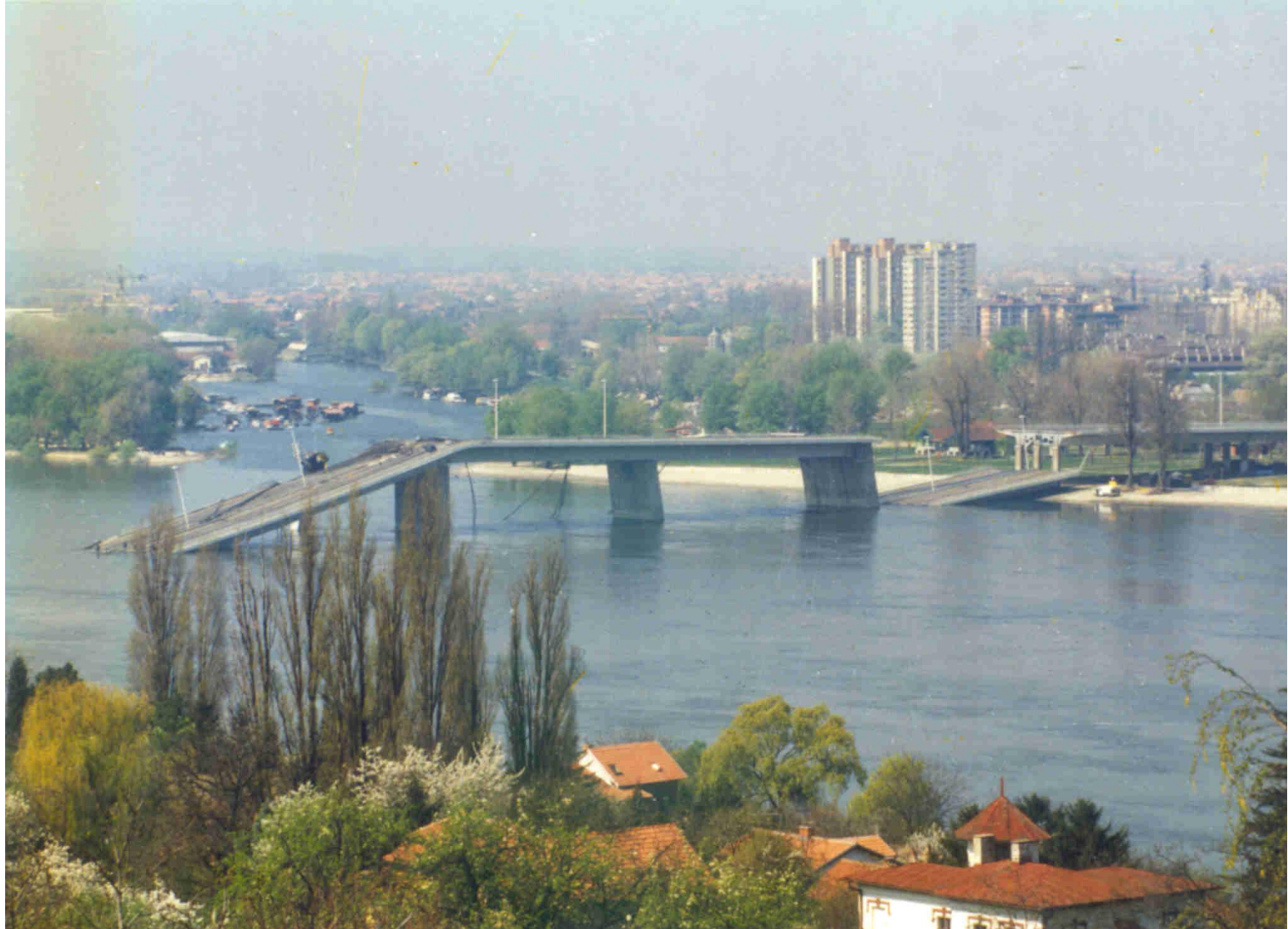
The Destruction of the Bridge Structure from the Left (Novi Sad) Side
