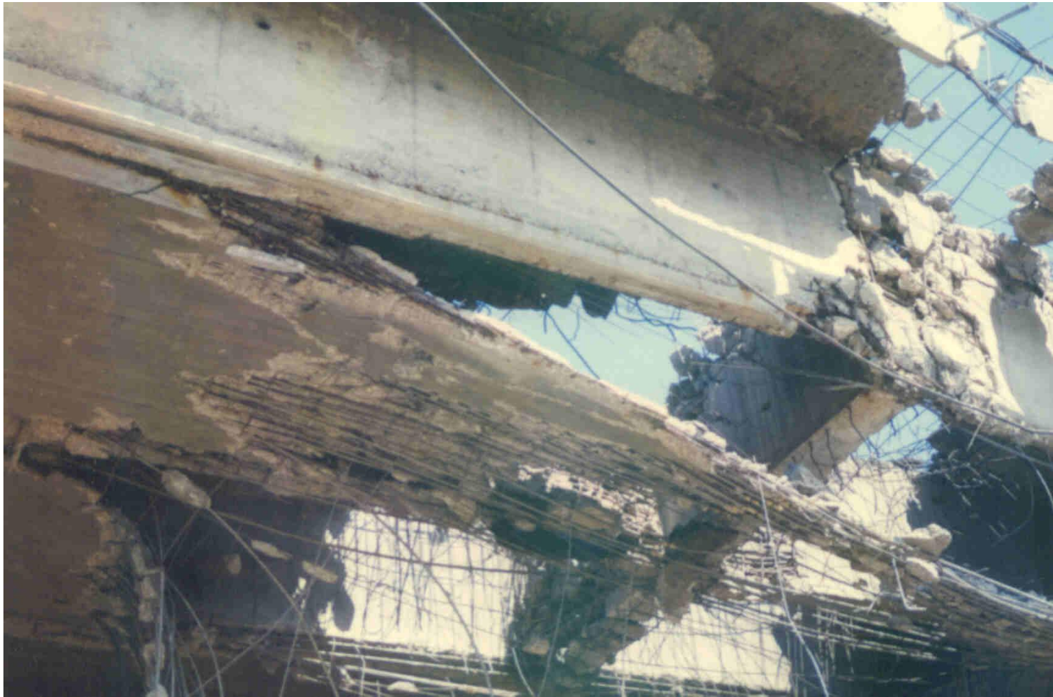
The Sight of the Damaged Deck Structure from the Bottom Side
