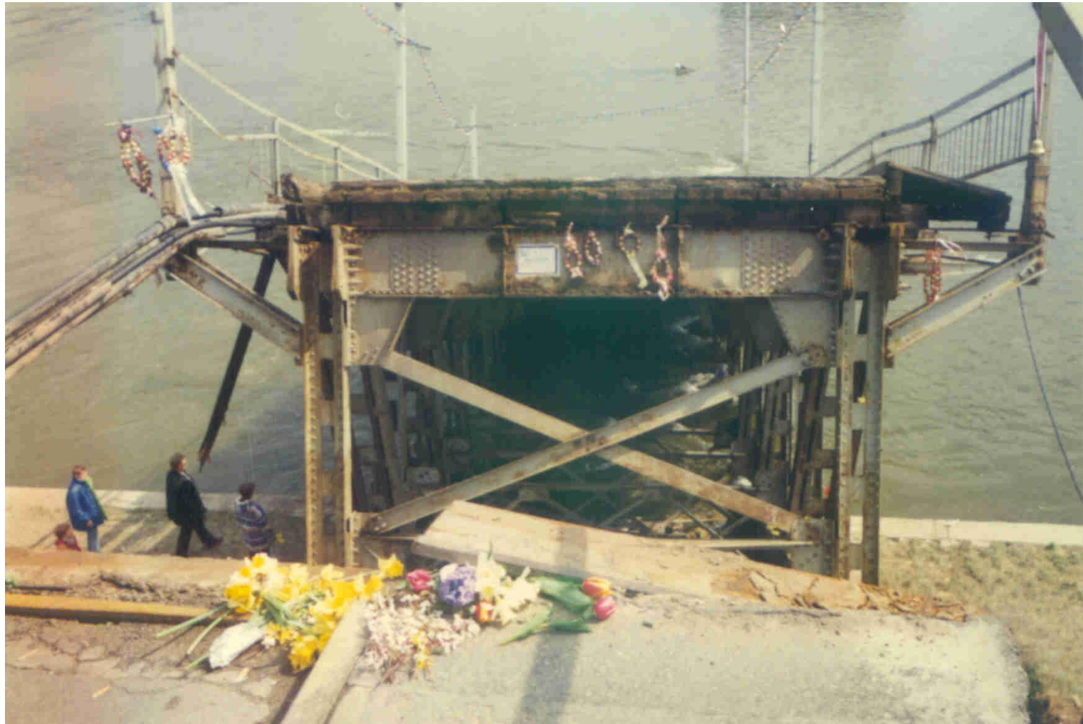
Ruins of the Inundation Structure of Varadin Bridge on Novi Sad Side
