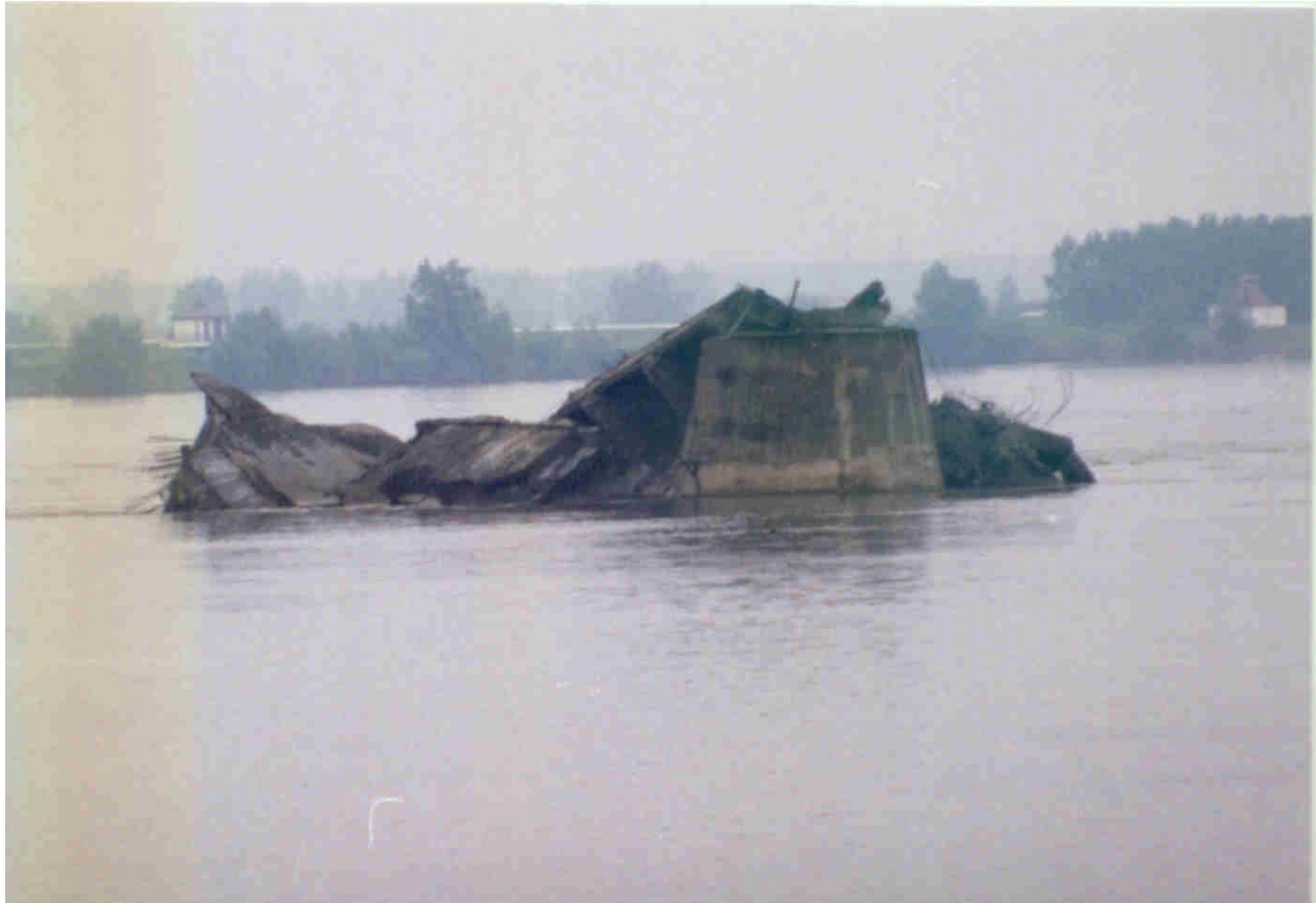
The Ruins of the Bridge near Middle Pier
