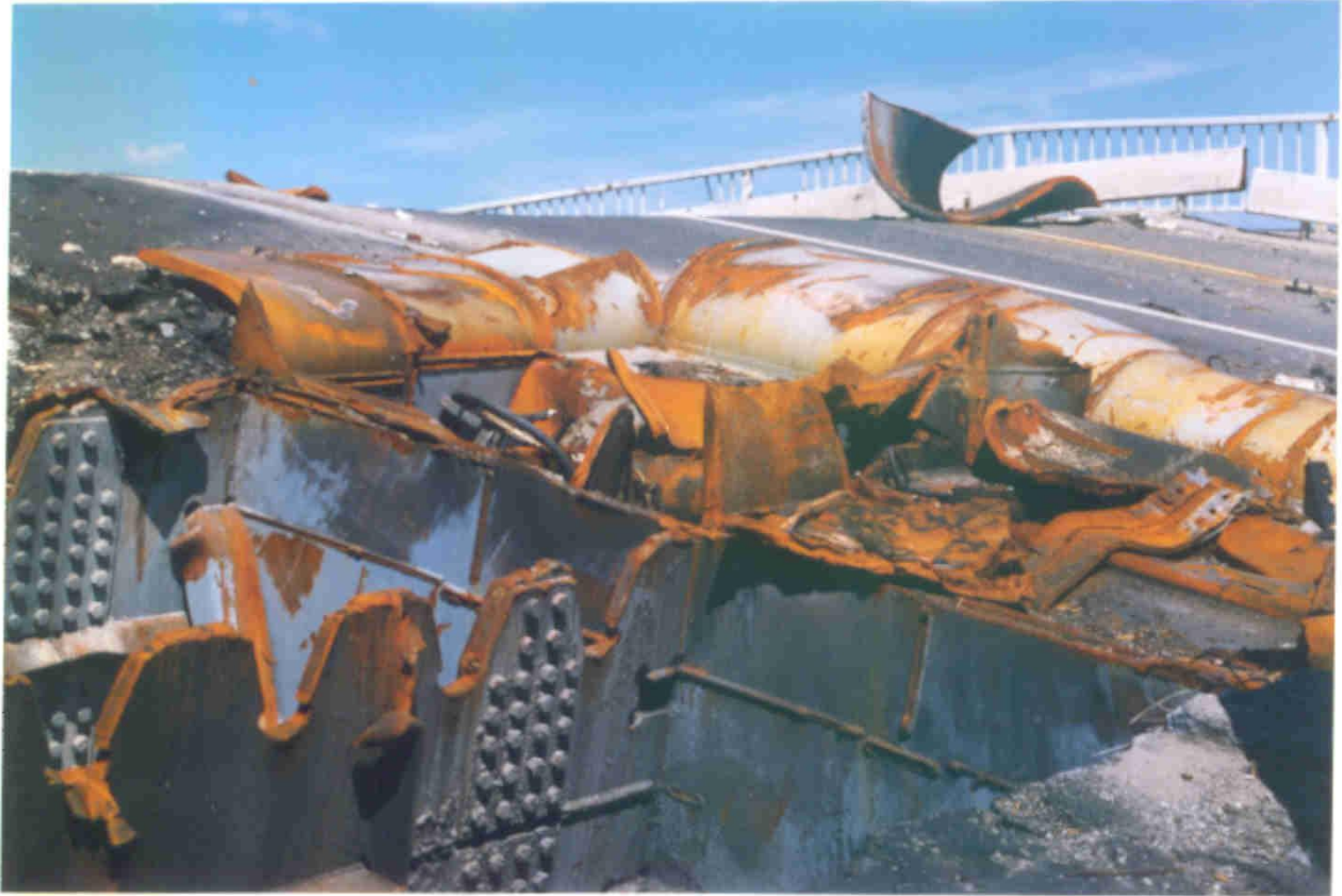
A Detail of the Broken Link Between the Pylon and Deck Structure
